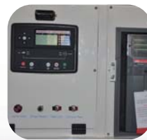
Control Panel & MCB
